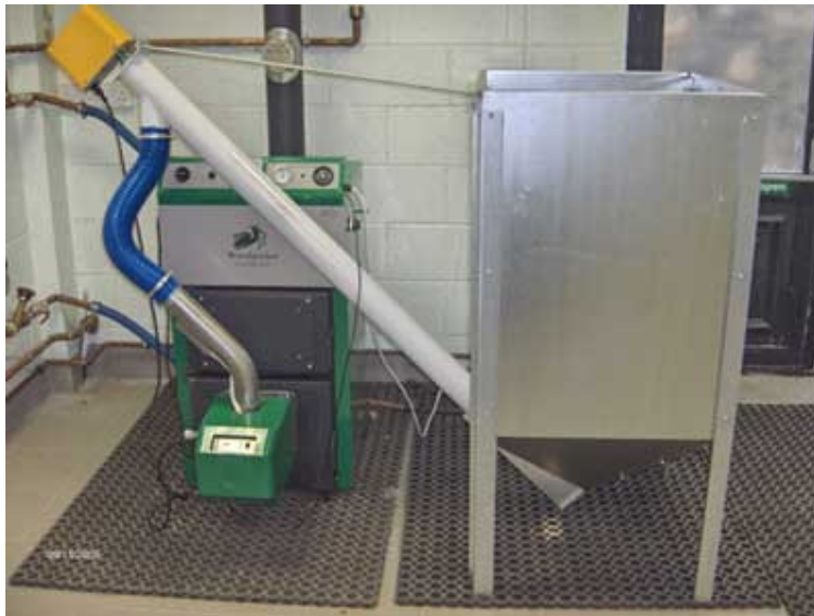
The Gerkross Wood Pellet Boiler
